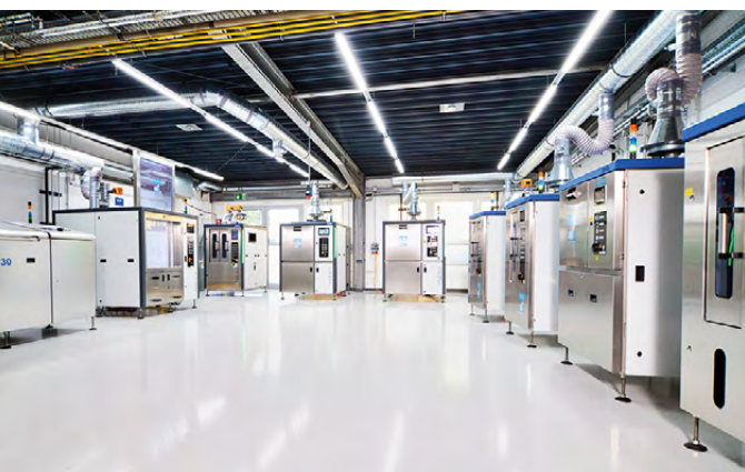
Technical centre of kolb Cleaning Technology GmbH in Willich
